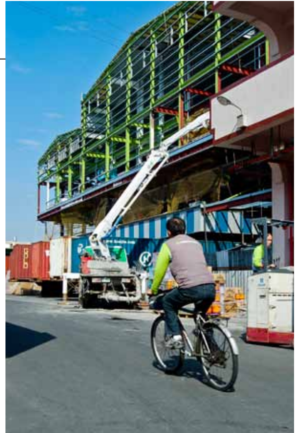
Merida's new paint factory, now under construction, is scheduled to open in March.
